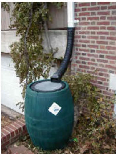
Figur 10. Regntønne for takvann. (District of Columbia Water & Sewer Authority)
